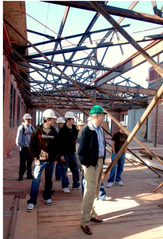
The San Francisco 2 team checking out the renovations at Ghirardelli Square. Hope they scored some chocolate!!
